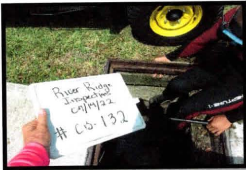
Need to Hydro cement this box to seal it proper
