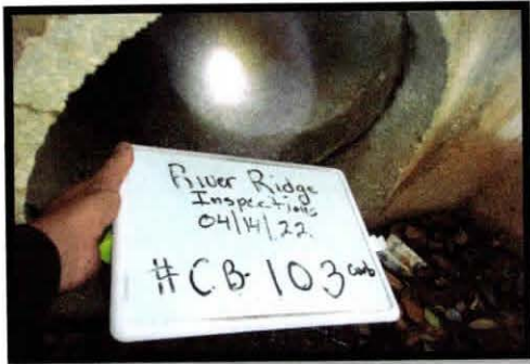
Pipe has crack recommend relining this pipe
