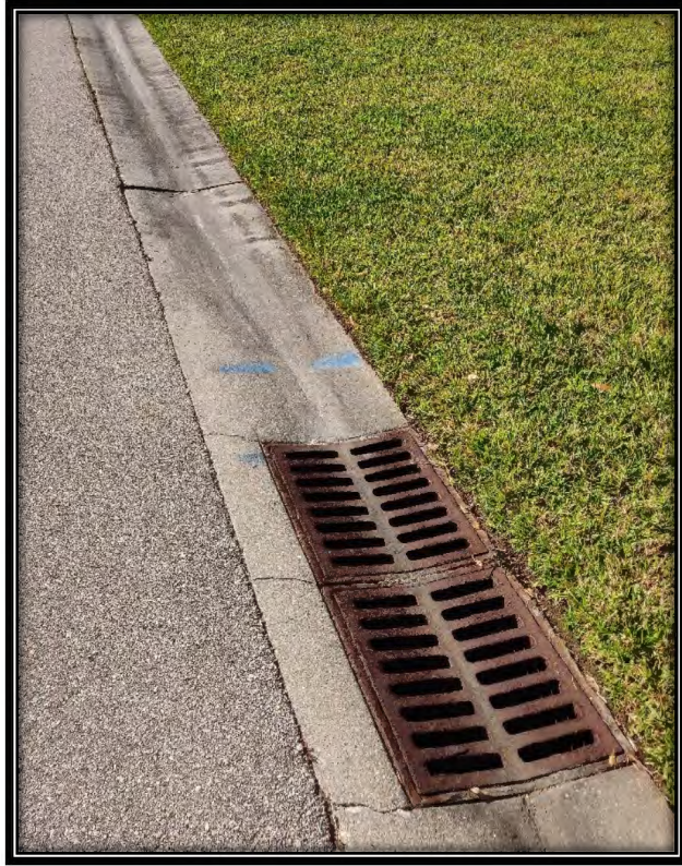
Figure 2: Minor obstruction and cracks in curb near inlet at 4518 Pinehurst Greens Ct
