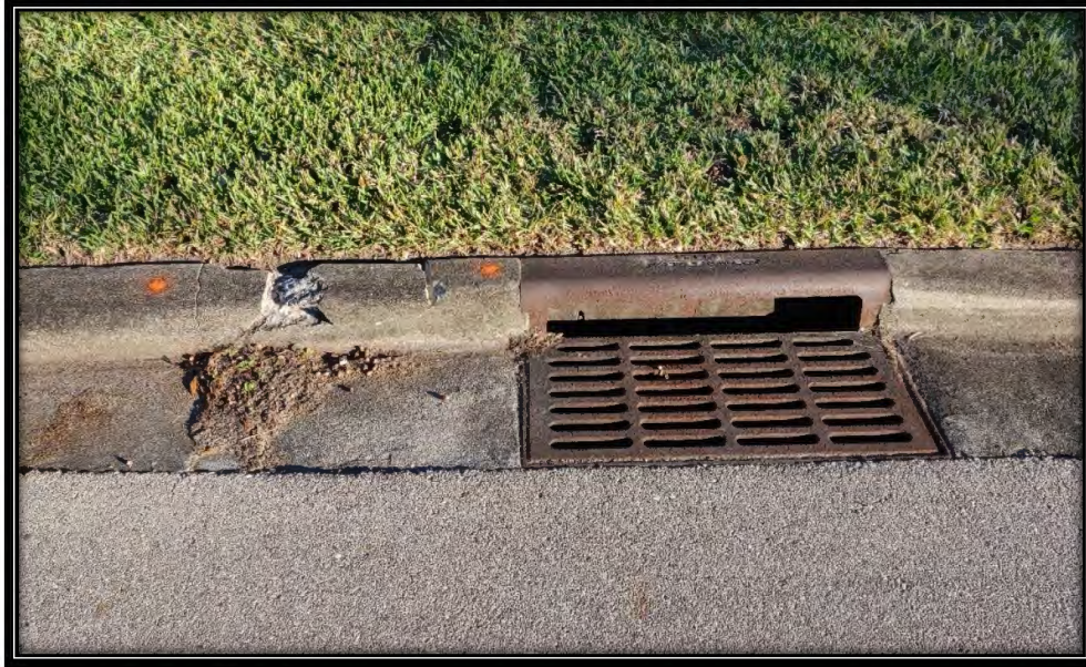
Figure 26: Large chip in curb on Pelican Sound Blvd., near Torrey Pines Way. Recommended ~3LF replacement
