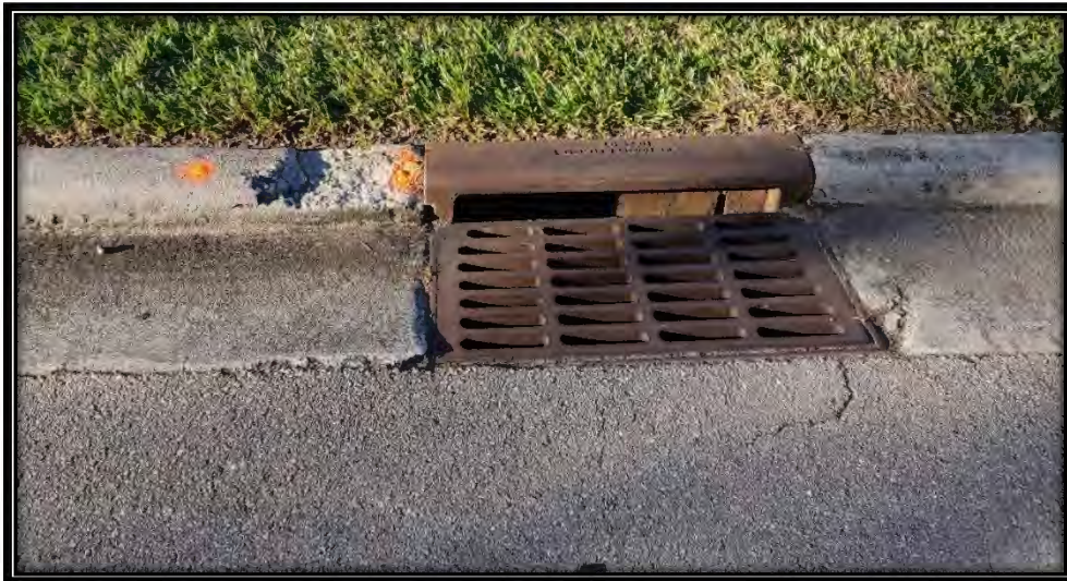
Figure 22: Large chip in curb at inlet on Pelican Sound Blvd. across from Golf Club, recommended ~3LF replacement each side of inlet
