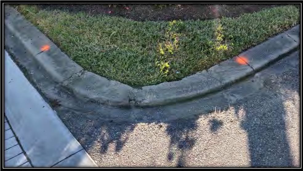
Figure 19: Moderate cracking in curb at Pinehurst Greens Ct. entrance, recommended ~8LF replacement
