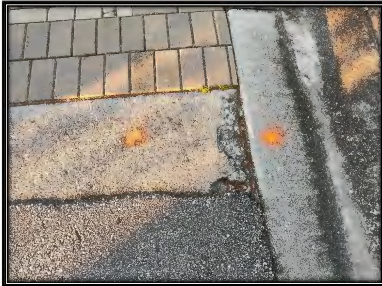
Figure 40: Moderate cracking in header curb at Southern Hills Dr. entrance, recommended ~2LF replacement
