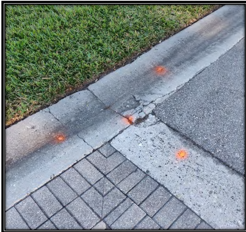
Figure 29: Major chips in valley gutter and header curb at Classics Court entrance, recommended replace ~4LF valley gutter & ~2LF header curb
