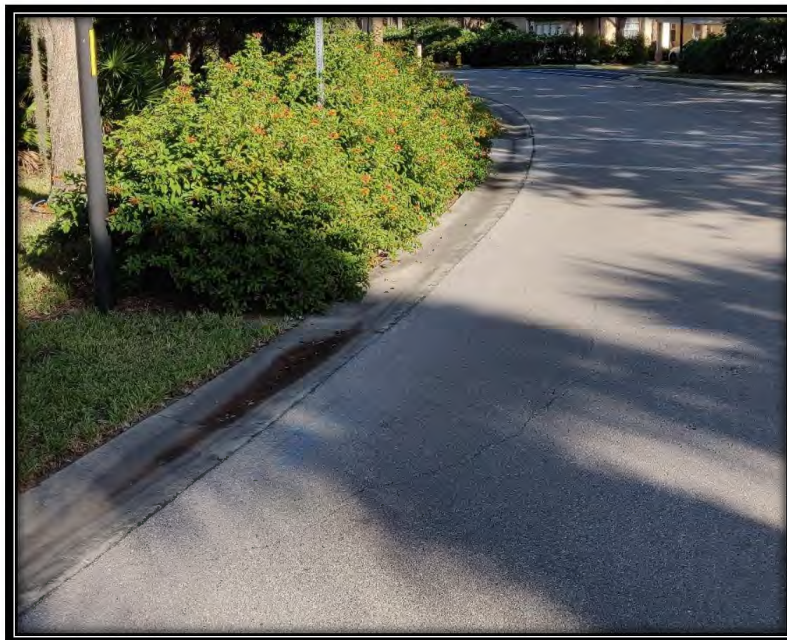
Figure 47: Slight cracks in pavement on Island Sound Cir. west of Pelican Sound Blvd.
