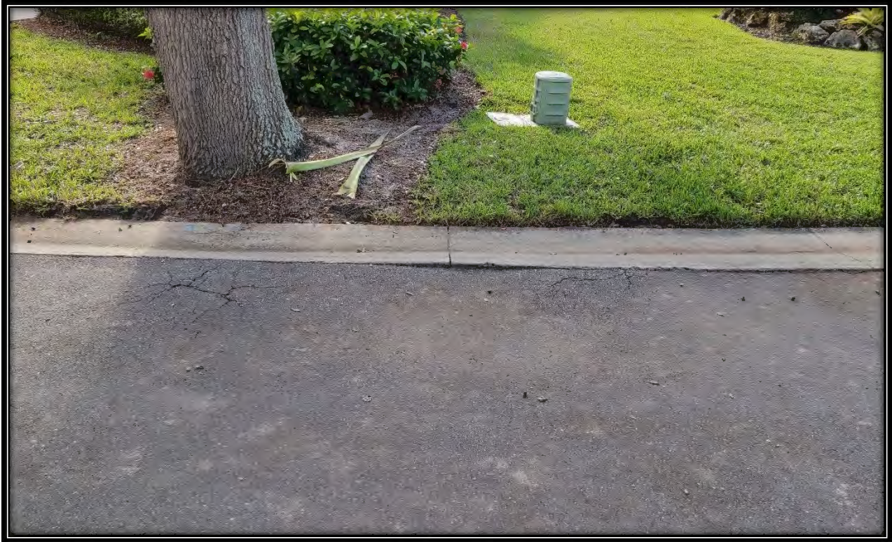
Figure 67: Raised asphalt and cracks from tree roots at 20816 Pinehurst Greens Dr.
