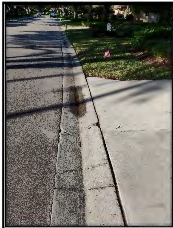
Figure 13: Minor cracks in curb at 21795 Sound Way
