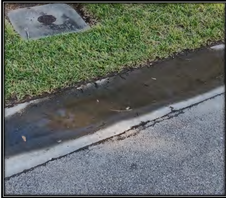
Figure 12: Minor cracks and ponding in curb at 21795 Sound Way
