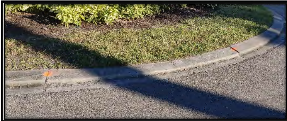
Figure 21: Settlement of curb in cul-de-sac island of Pinehurst Greens Ct., with moderate obstruction. Recommended ~10LF replacement
