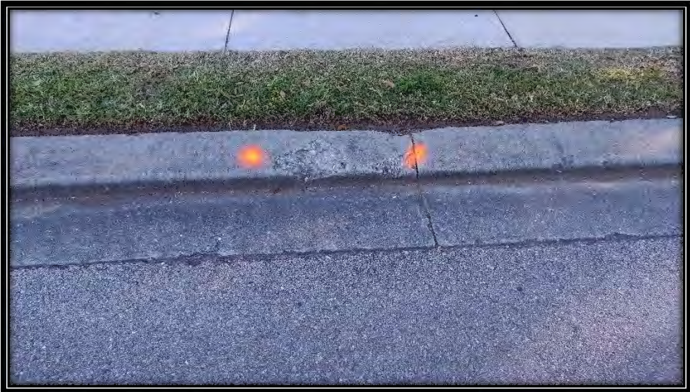
Figure 18: Large chip in curb face at Pelican Sound Blvd. east of Golf Club, recommended ~2LF replacement
