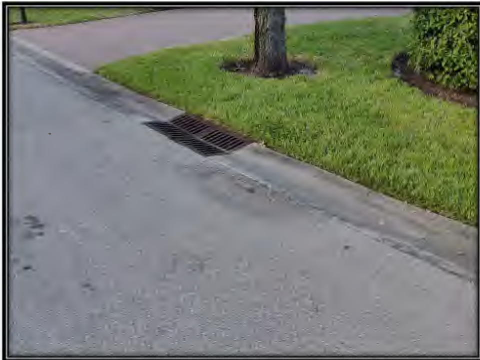
Figure 62: Asphalt cracks and signs of settlement at 21825 Masters Circle
