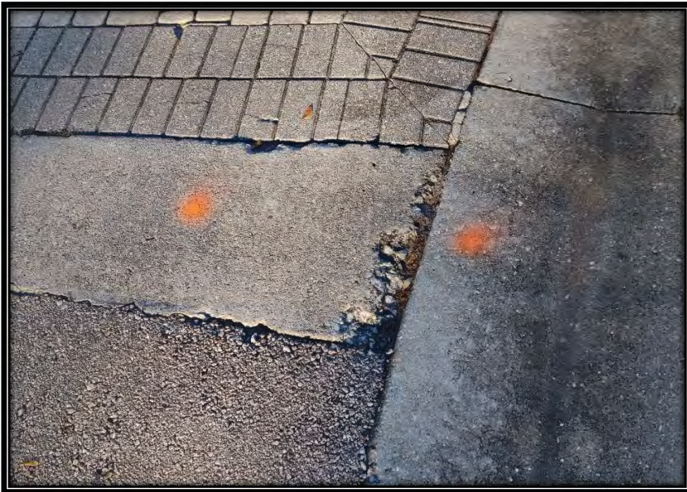
Figure 31: Large chip in header curb on Palmetto Dunes Dr. at Classics Ct. entrance, recommended ~2LF replacement
