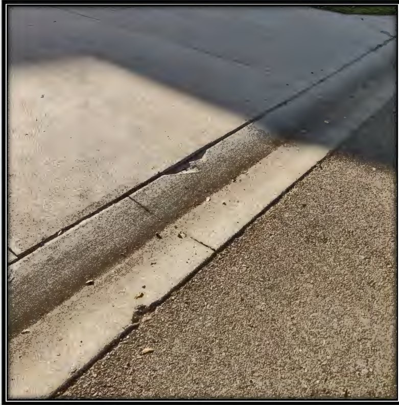
Figure 10: Minor curb chips at 21770 Palmetto Dunes Dr.
