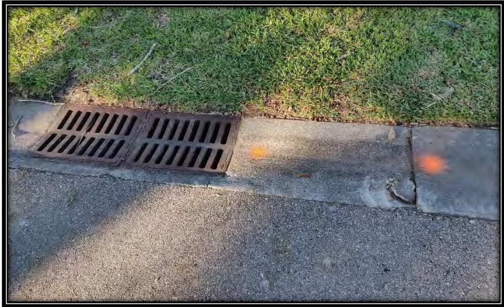
Figure 24: Moderate obstruction in curb next to 20859 Gleneagles Links Dr., recommended ~2LF replacement, right side of inlet
