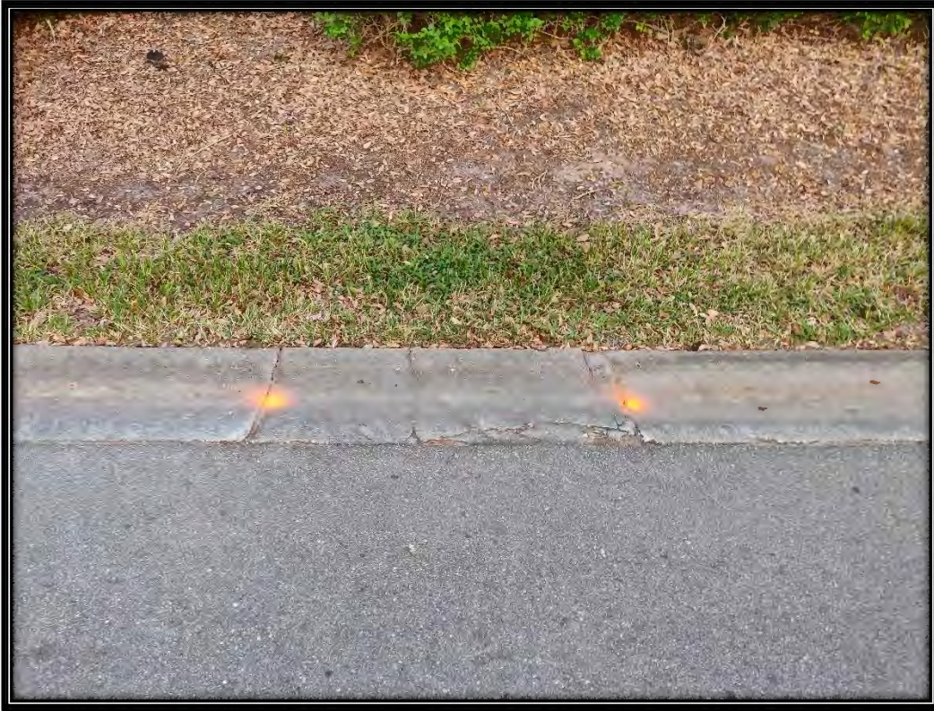
Figure 42: Moderate cracking in curb on Pelican Sound Dr. near Sound Way intersection, recommended ~4LF replacement
