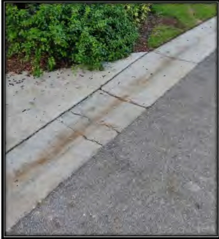
Figure 16: Minor curb cracks at dumpster enclosure on Southern Hills Dr.
