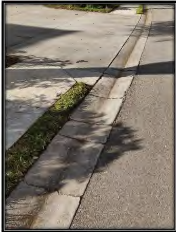
Figure 6: Minor cracks in curb at 21340 Pelican Sound Dr.
