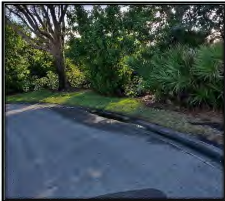
Figure 5: Water ponding in curb in west side of Torrey Pines Way cul-de-sac
