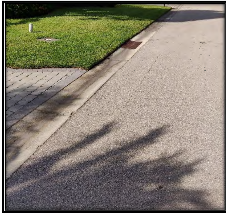
Figure 53: Potential settlement of asphalt and curb at 20832 Pinehurst Greens Dr.
