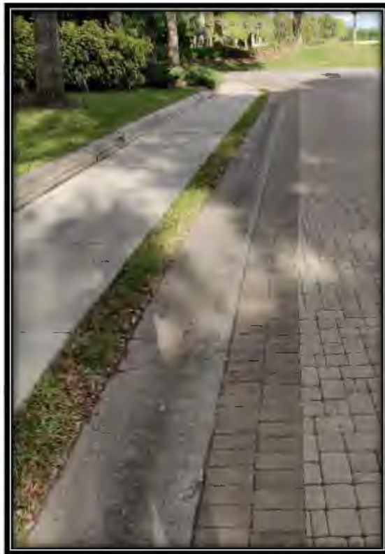
Figure 7: Minor cracks in curb on north side of Sound Way at intersection with Pelican Sound Blvd.
