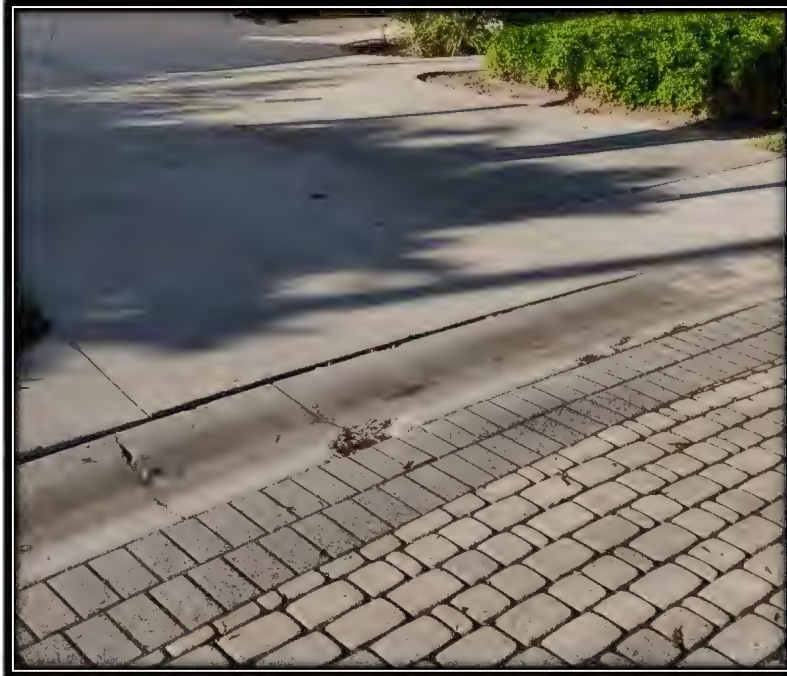
Figure 32: Moderate curb chips at 7851 Classics Ct., recommended ~4LF replacement
