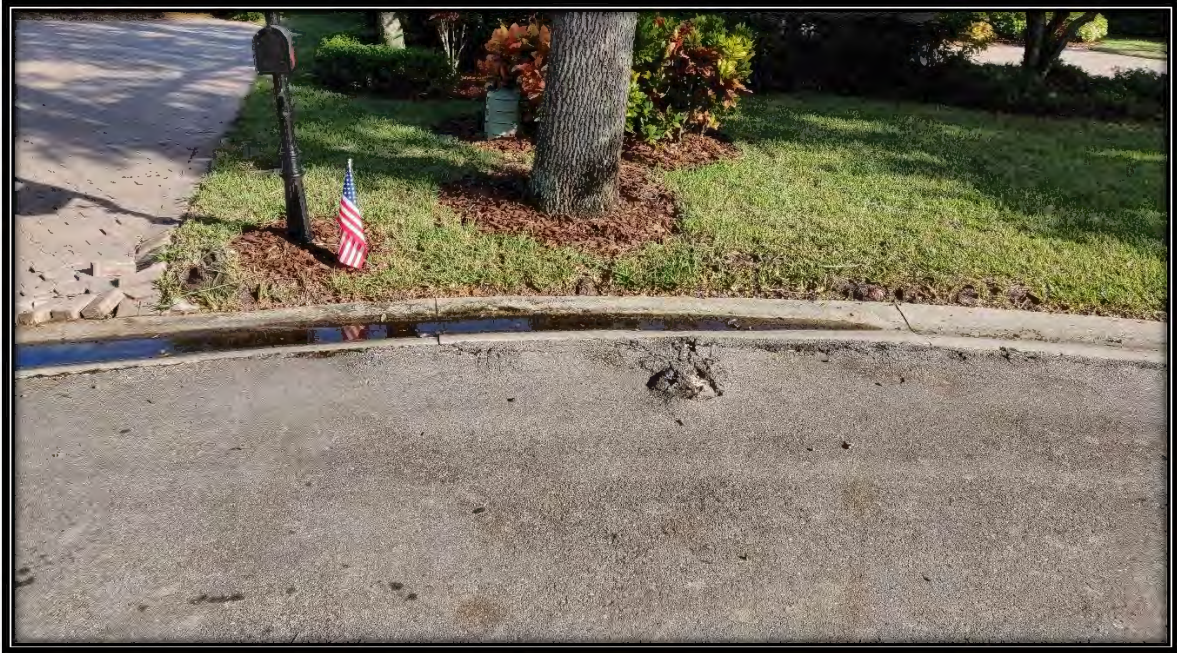
Figure 70: Significant pavement damage and damages to nearby curb and pavers at 20781 Torrey Pines Way
