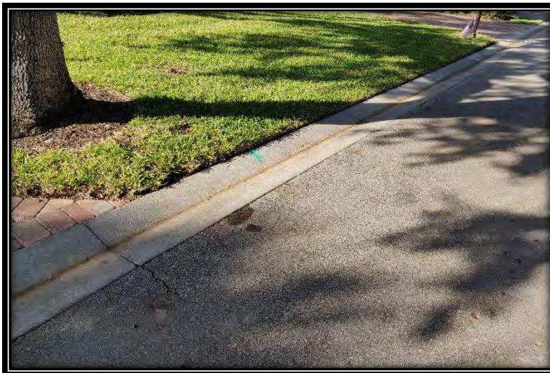
Figure 45: Slight cracks and stains in pavement at 20858 Gleneagles Links Dr.
