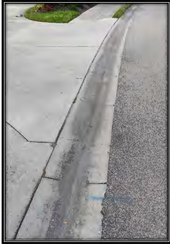
Figure 8: Minor curb cracks in side entrance to 21841 Palmetto Dunes Dr.
