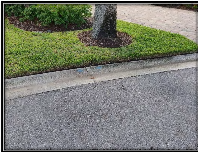
Figure 69: Minor cracks in asphalt near tree at 4631 Gleneagles Links Ct.
