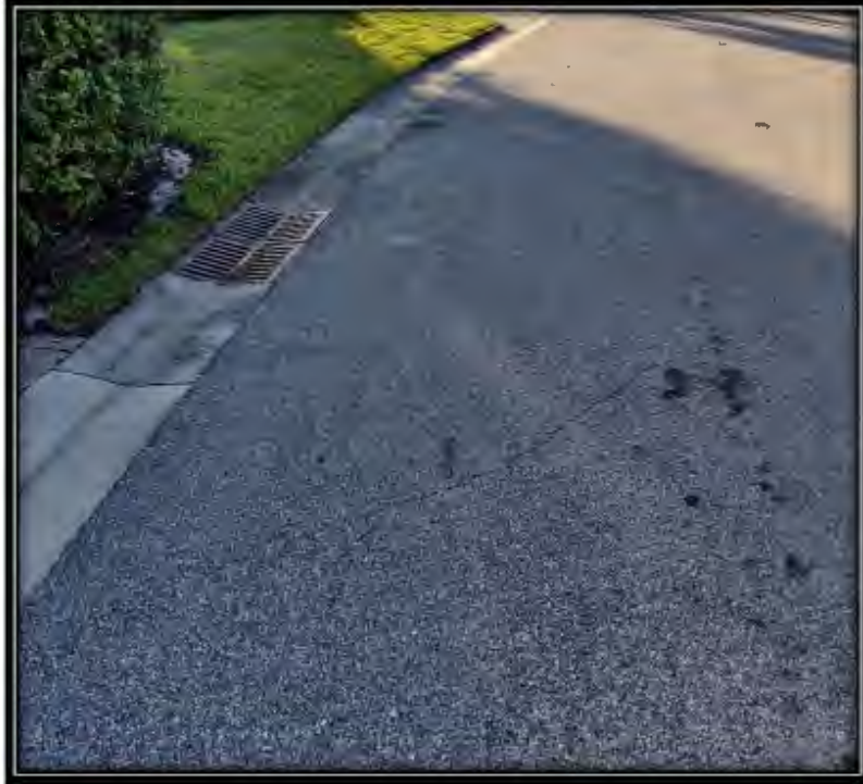
Figure 61: Asphalt cracks and signs of settlement at 21832 Masters Circle
