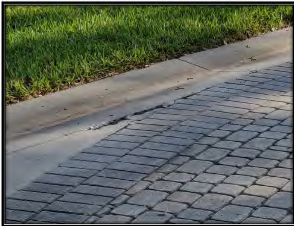
Figure 33: Moderate crushing of header curb in front of 7850 Classics Ct., recommended ~2LF replacement
