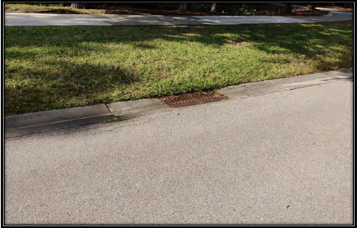
Figure 55: Asphalt cracks and signs of settlement at inlet across from 20921 Pinehurst Greens Drive
