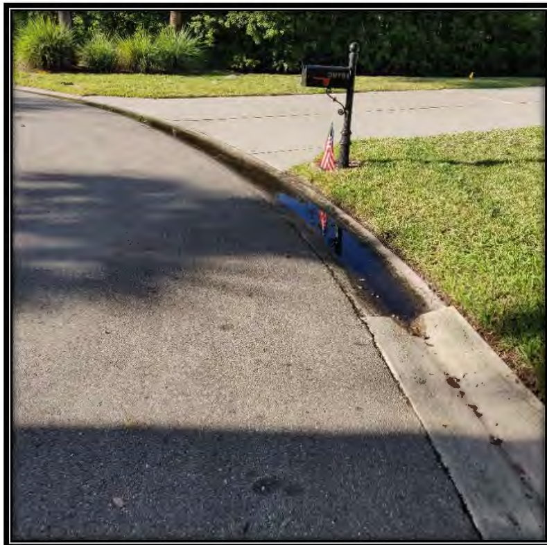
Figure 71: Water ponding in curb due to low point caused by damages at 20781 Torrey Pines Way
