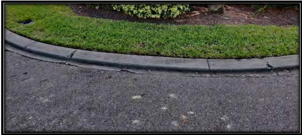
Figure 25: Moderate curb cracks and chips in Gleneagles Links Dr. cul-de-sac island, recommended ~10 LF replacement
