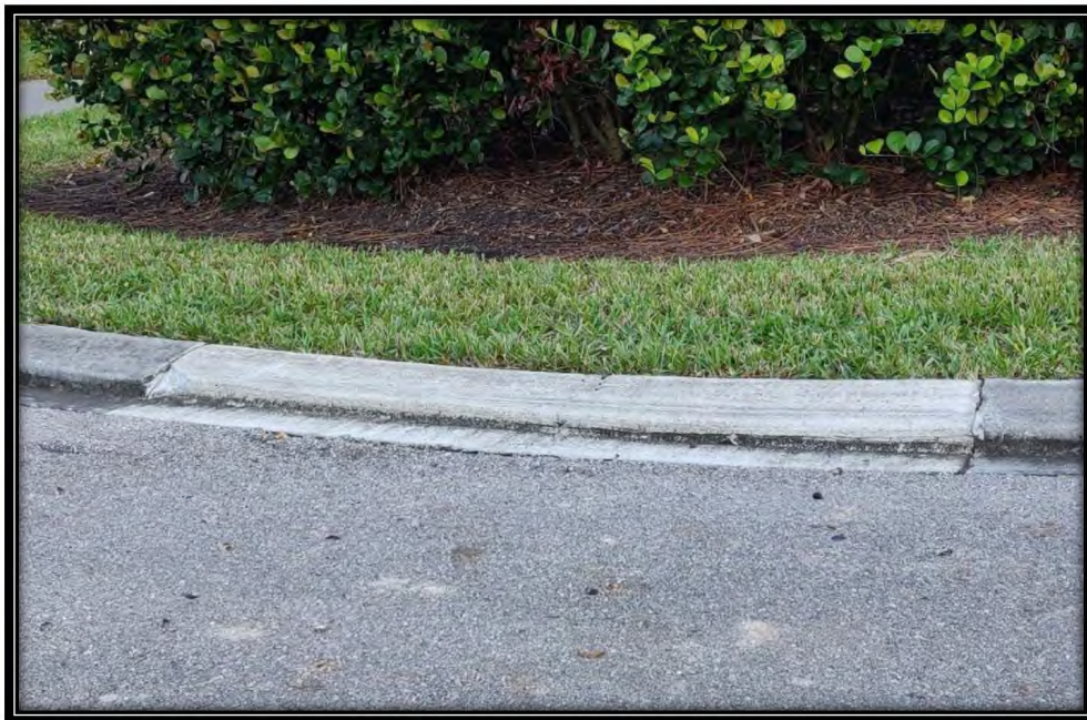
Figure 3: Minor settlement of previous curb replacement in Gleneagles Links Dr. cul-de-sac island
