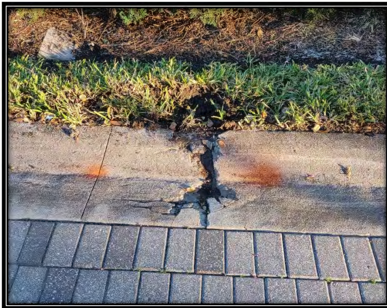
Figure 43: Moderate cracking in curb at Masters Circle entrance, recommended ~2LF replacement
