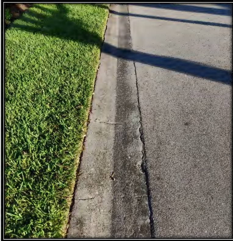
Figure 14: Minor curb cracks at 21916 Masters Circle
