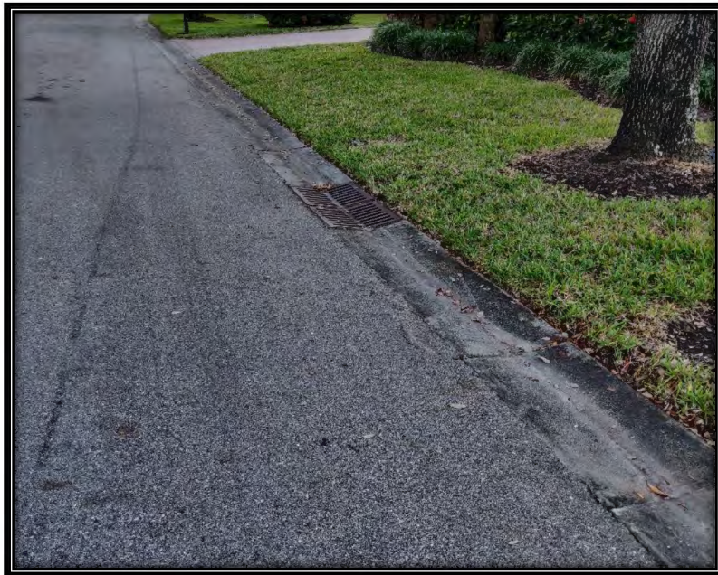
Figure 64: Minor asphalt damage around inlet at 21863 Masters Circle
