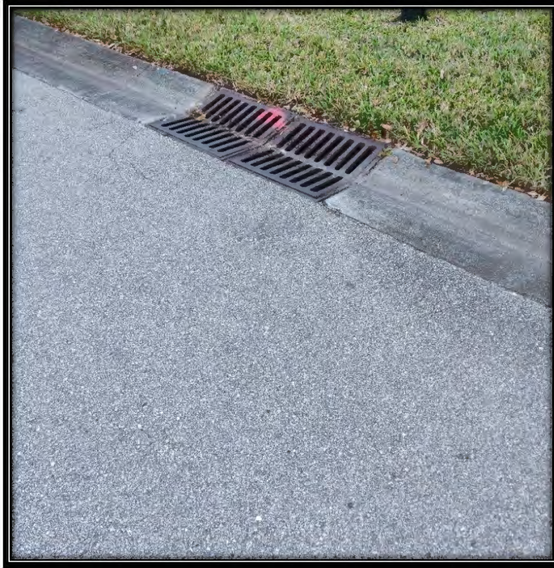
Figure 65: Minor settlement and asphalt cracks around inlet at 21864 Masters Circle
