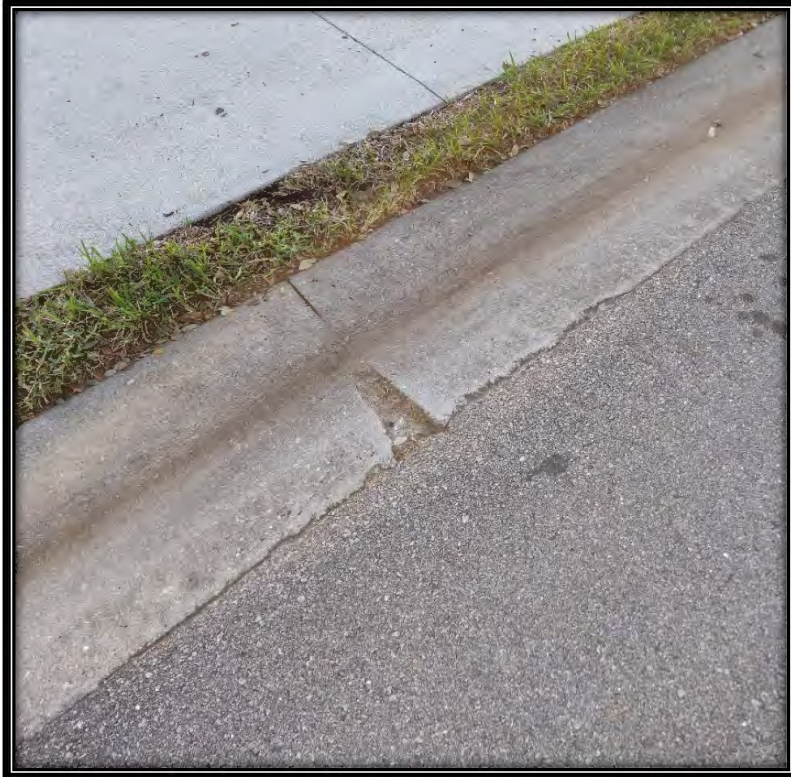
Figure 36: Moderate chip in curb at 21450 Pelican Sound Dr., recommended ~2LF replacement
