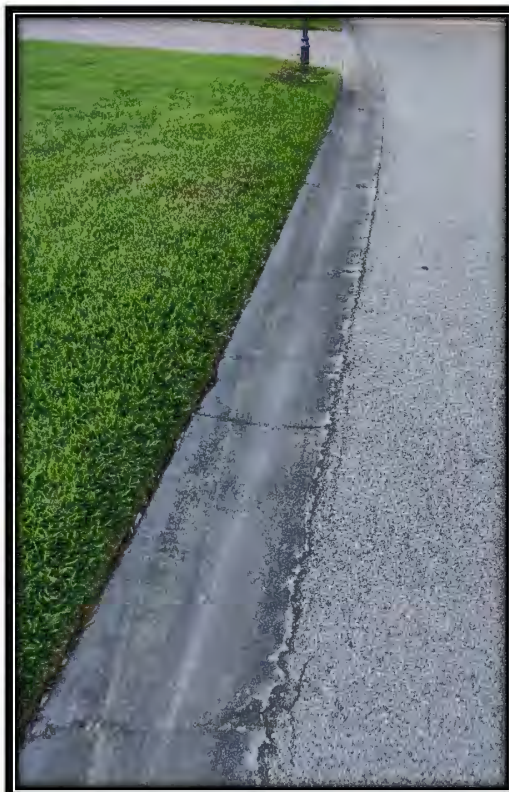
Figure 15: Minor curb cracks and raveling at 21895 Masters Circle
