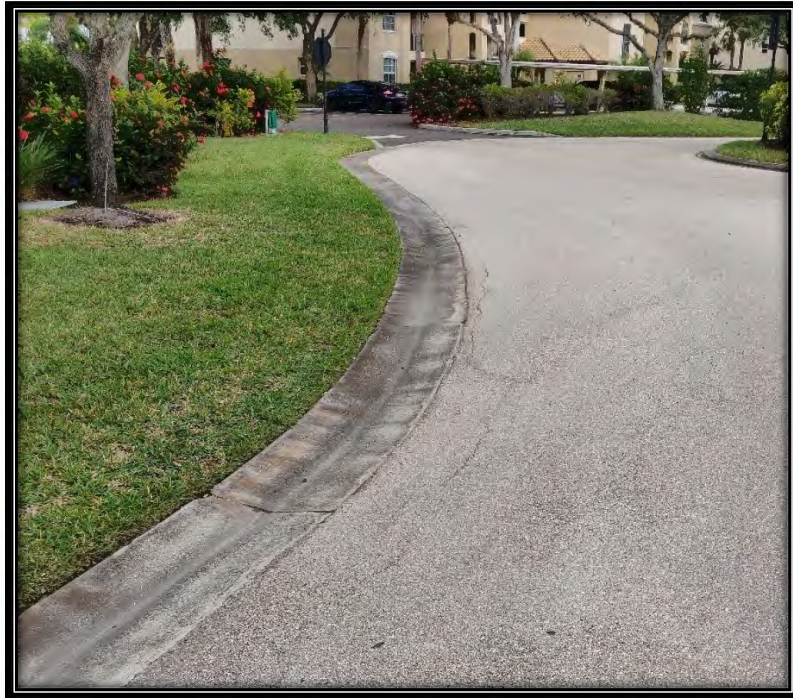
Figure 49: Minor cracks in pavement on Turnberry Lake Dr. roundabout near 4670 Turnberry Lake Dr.
