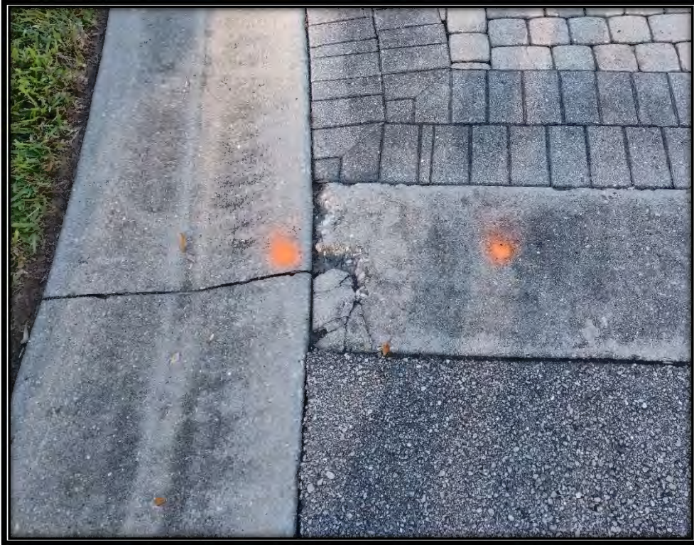
Figure 30: Moderate cracking in header curb at Classics Ct. entrance, recommended ~2LF replacement at each end of header curb
