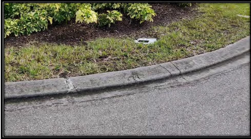
Figure 20: Moderate cracking in curb at Pinehurst Greens Ct. cul-de-sac, recommended ~5LF replacement
