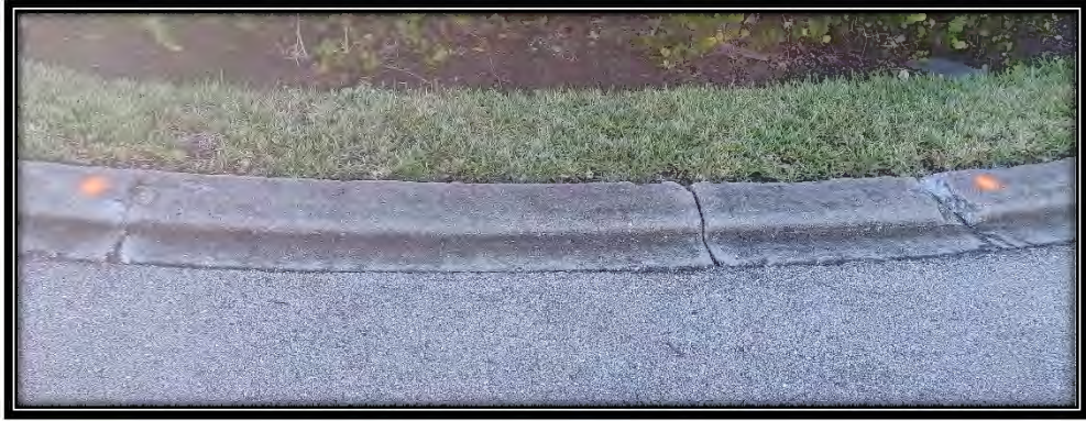
Figure 23: Moderate cracking in curb at cul-de-sac island of Gleneagles Links Ct., recommended ~10LF replacement
