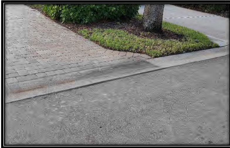
Figure 44: Slight settlement and water damage in pavement at 20824 Gleneagles Links Dr.
