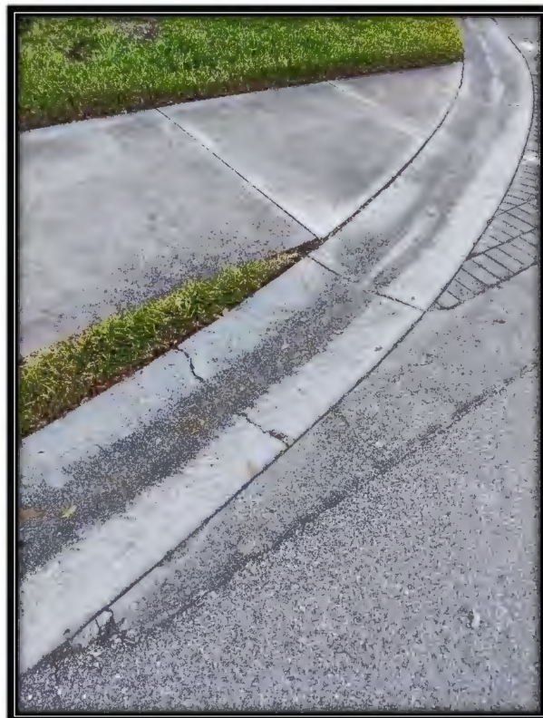
Figure 11: Minor cracks in curb at SW corner of intersection of Palmetto Dunes Dr. and Sound Way
