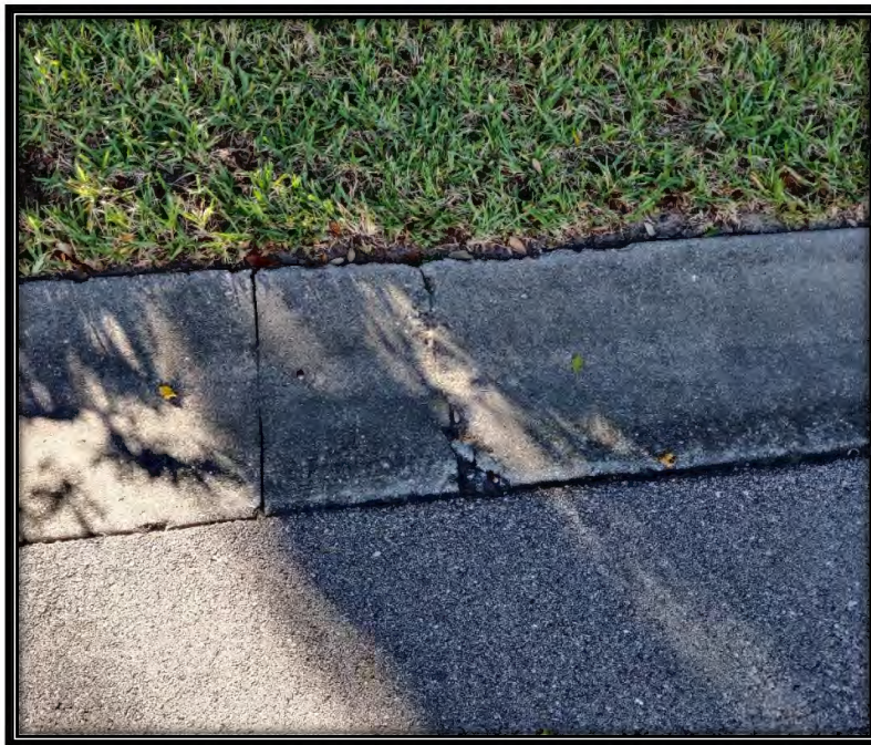
Figure 27: Moderate crack in curb across street from 20925 Island Sound Cir., recommended ~2LF replacement
