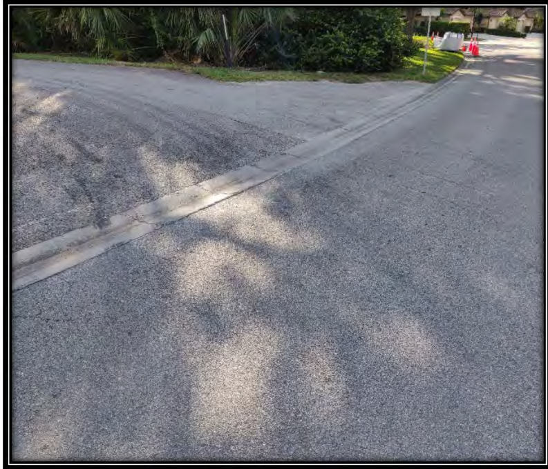
Figure 48: Surface wear in pavement on Island Sound Cir. at FPL Easement
