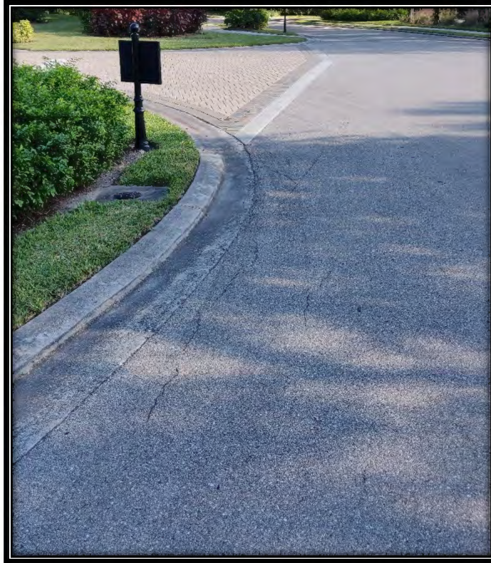
Figure 46: Slight cracks in pavement at entrance to Torrey Pines Way
