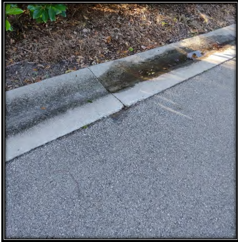
Figure 52: Small chip in pavement at entrance to Southern Hills Dr.
