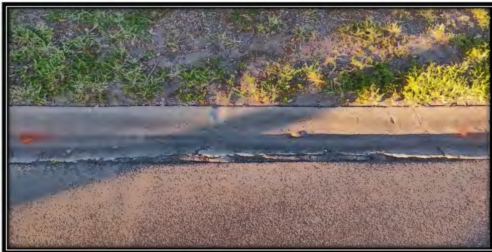
Figure 41: Moderate cracking in curb on Pelican Sound Dr. near 21521 Pelican Sound Dr., recommended ~10LF replacement
