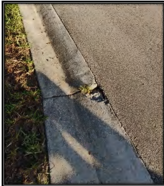
Figure 39: Moderate curb chip on Southern Hills Ct. at intersection with Southern Hills Dr., recommended ~2LF replacement
