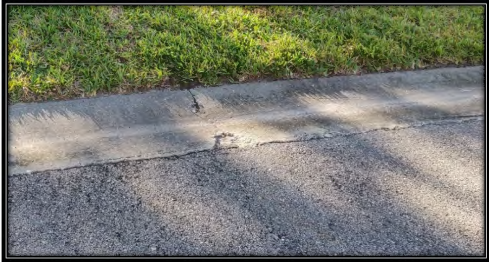
Figure 28: Miderate chipping in curb on west side of roadway south of T-intersection of Island Sound Cir., recommended ~2LF replacement
