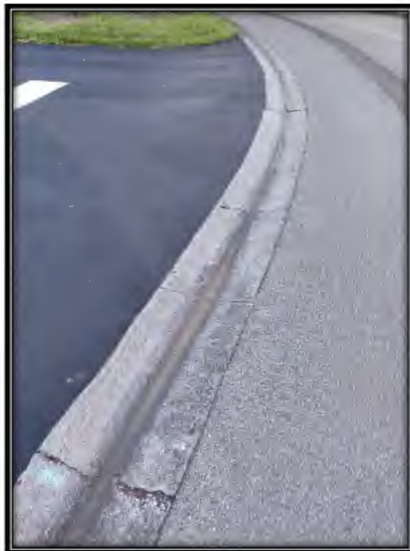
Figure 17: Minor curb cracks on Pelican Sound Dr. at intersection with Pelican Sound Blvd.
