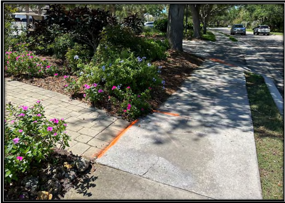
Figure 16: Cracked and raised sidewalk panel along Pelican Sound BLVD Near east parking lot entrance to Clubhouse.
