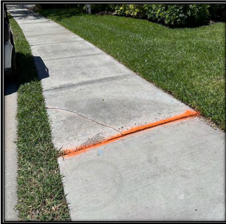
Figure 18: Raised and cracked sidewalk panel and transition at 21410 Pelican Sound Drive.
