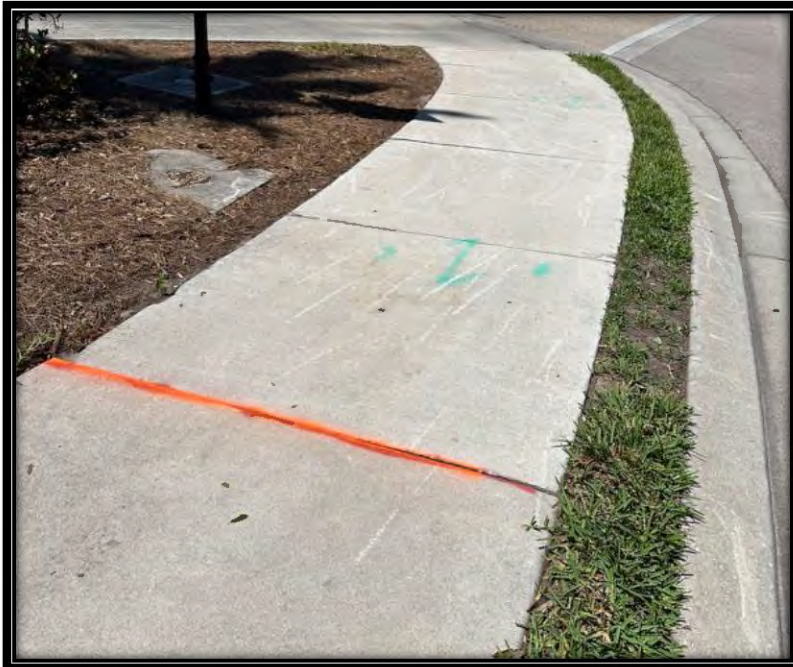
Figure 6: Raised sidewalk transition at intersection of Seaside Edgewater and Pelican Sound BLVD.
