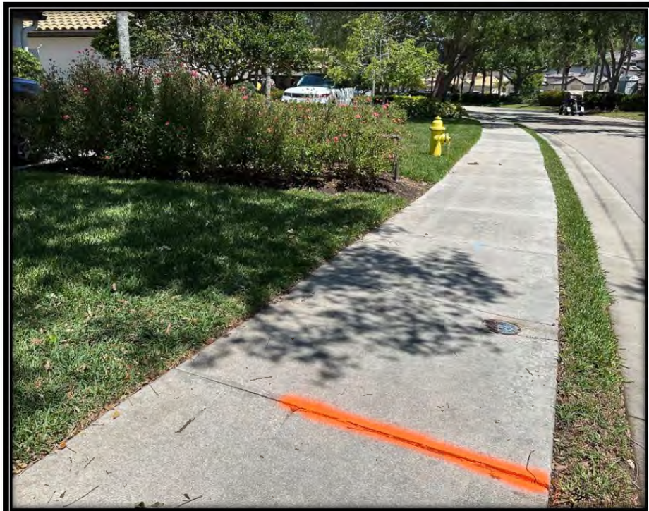
Figure 9: Raised sidewalk transition at 21380 Pelican Sound Drive.
