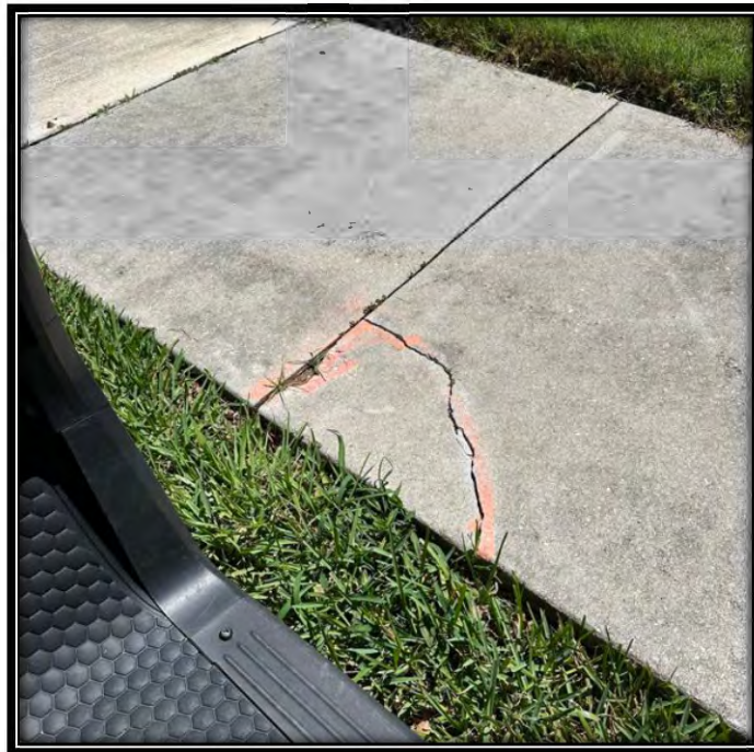
Figure 22: Cracks in sidewalk and signs of settlement along Pelican Sound Drive between Masters Circle and Southern Hills Dr entrances.
