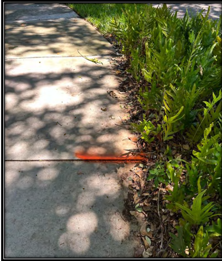
Figure 12: Raised sidewalk transition along Pelican Sound Drive across from Southern Hills Drive entrance.
