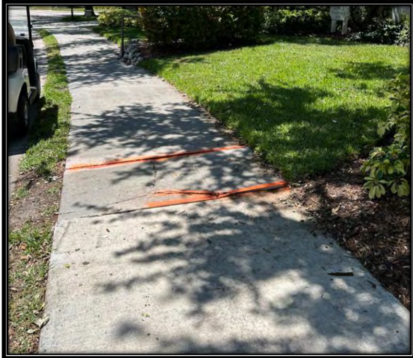
Figure 19: Raised and cracked sidewalk panel and transition at 21430 Pelican Sound Drive.
