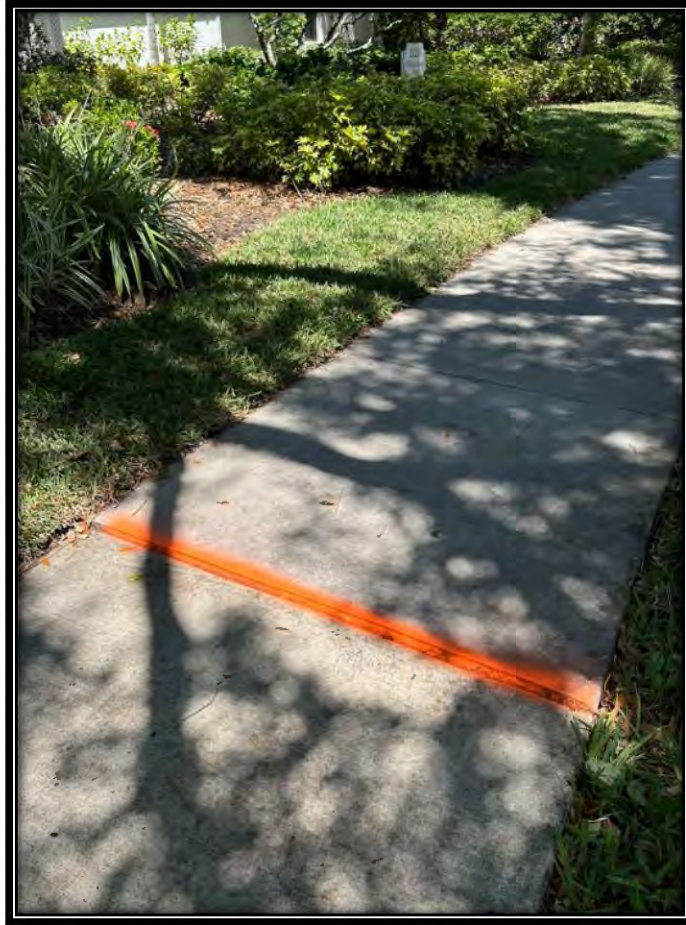
Figure 8: Raised sidewalk transition at 21210 Pelican Soud Drive.
