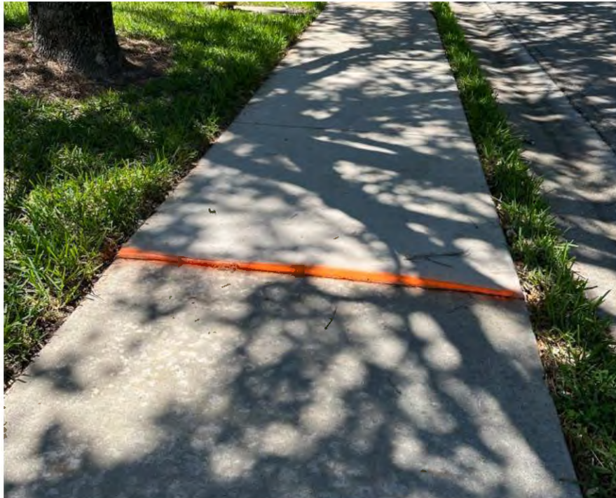
Figure 13: Raised sidewalk transition along Pelican Sound Drive between Masters Circle and Southern Hills Dr entrances.
