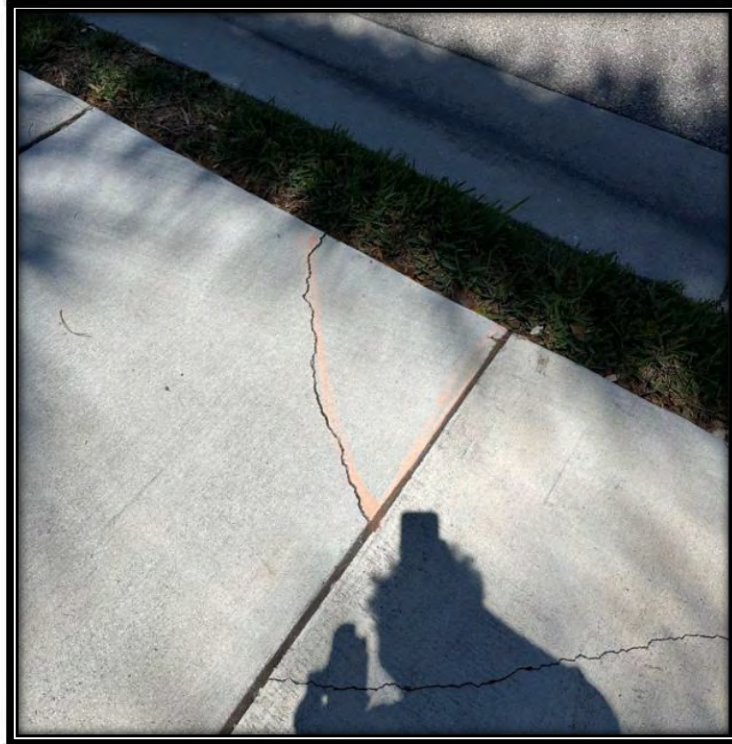
Figure 21: Cracks in sidewalk and signs of settlement at intersection of Masterc Circle and Pelican Sound Drive.
