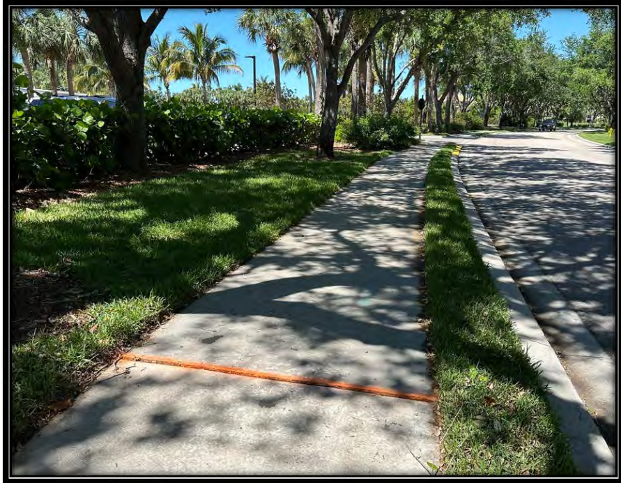
Figure 4: Raised sidewalk along Pelican Sound BLVD in front of west parking lot of Clubhouse.
