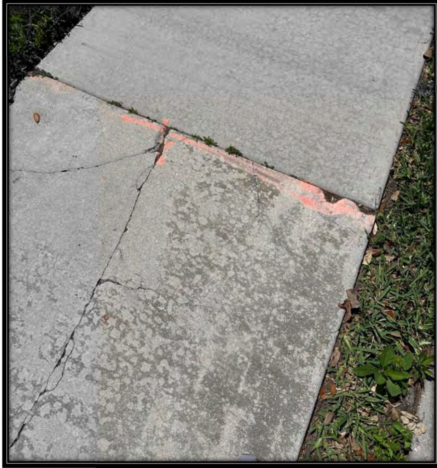
Figure 23: Cracks in sidewalk and signs of settlement along Pelican Sound Drive between Masters Circle and Southern Hills Dr entrances.
