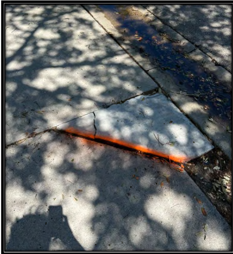
Figure 20: Raised and cracked sidewalk panel and transition at 21748 Pelican Sound Drive.
