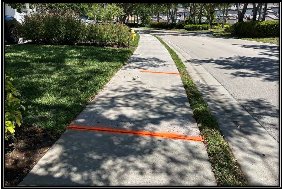
Figure 10: Raised sidewalk transition at 21380 Pelican Sound Drive.
