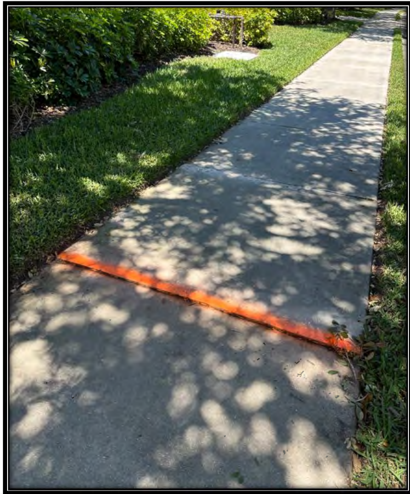
Figure 11: Raised sidewalk transition at 21726 Pelican Sound Drive.
