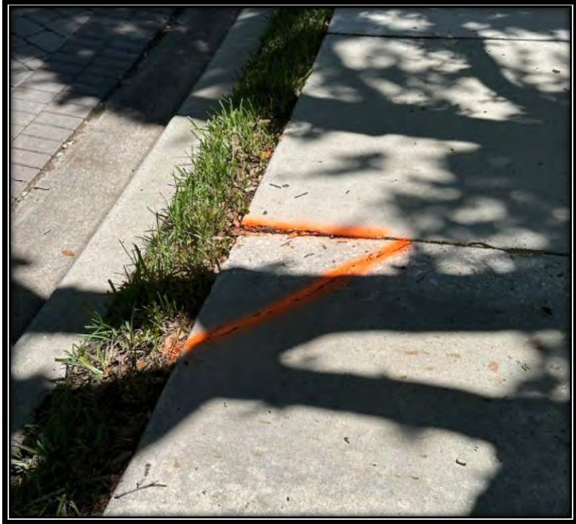
Figure 17: Raised and cracked sidewalk transition approaching roundabout and community entrance/exit on Pelican Sound BLVD.
