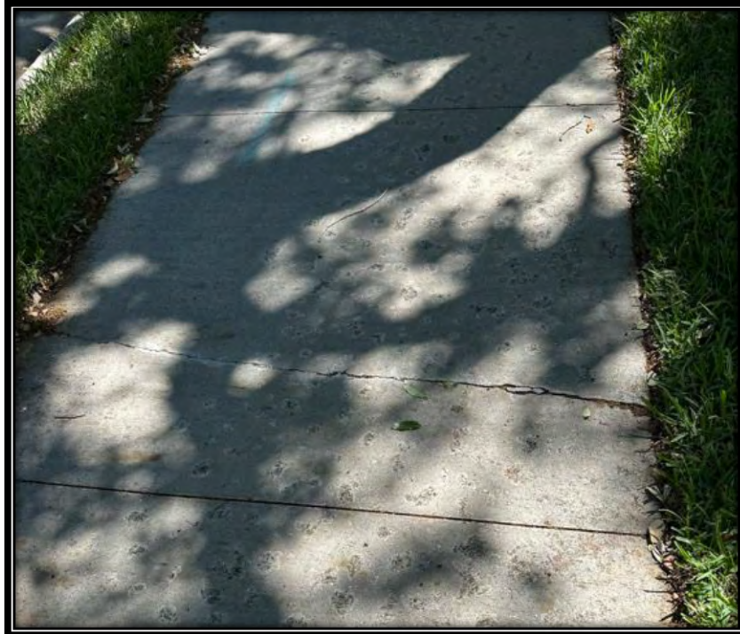
Figure 14: Cracked concrete panel along Pelican Sound BLVD in front of west parking lot of Clubhouse.
