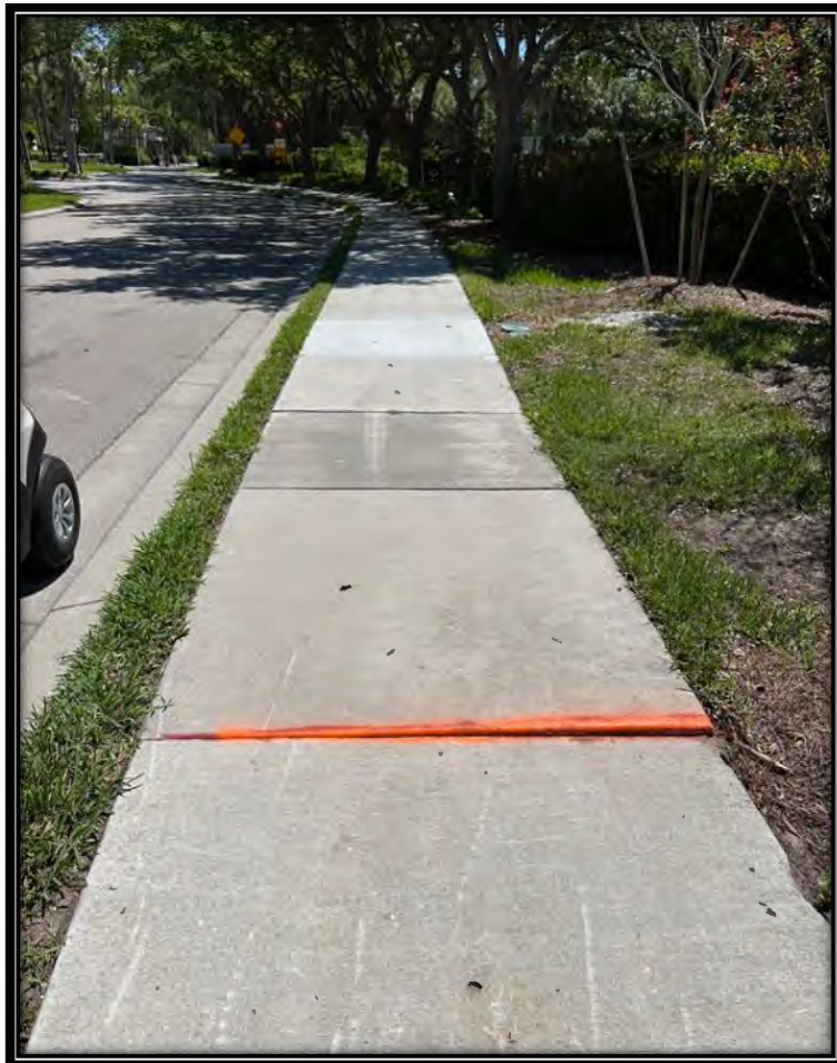
Figure 5: Raised sidewalk transition approaching roundabout and community entrance/exit on Pelican Sound BLVD
