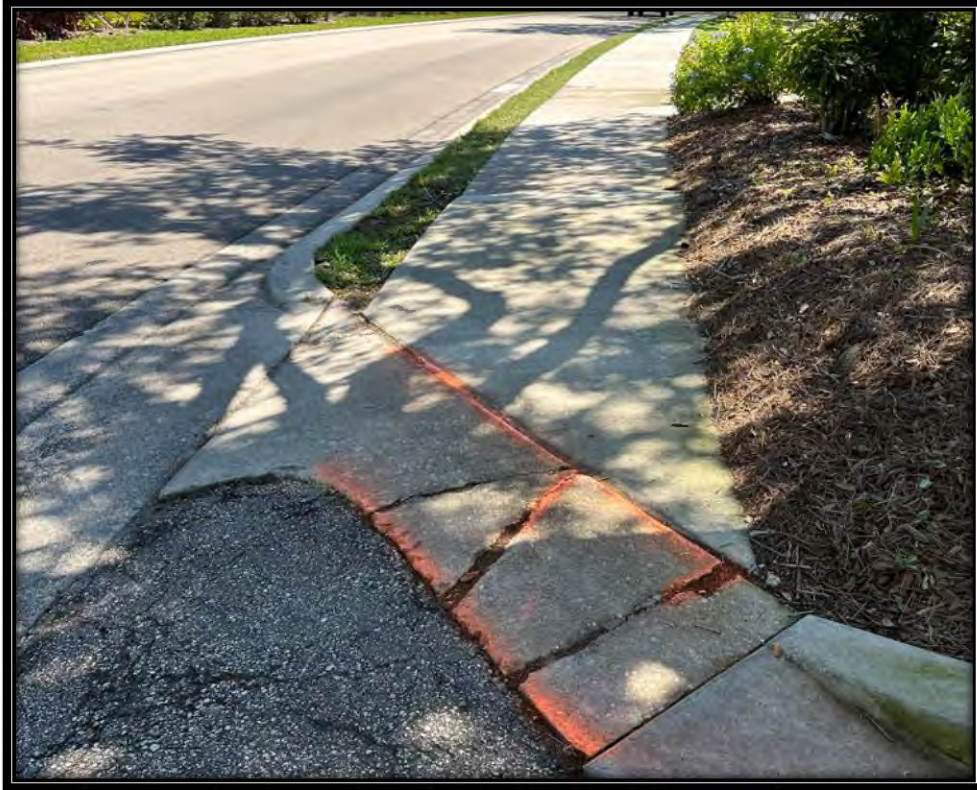
Figure 15: Cracked and raised sidewalk transition along Pelican Sound BLVD at east parking lot entrance to Clubhouse.
