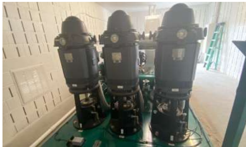
THE NEW PUMP SKID
